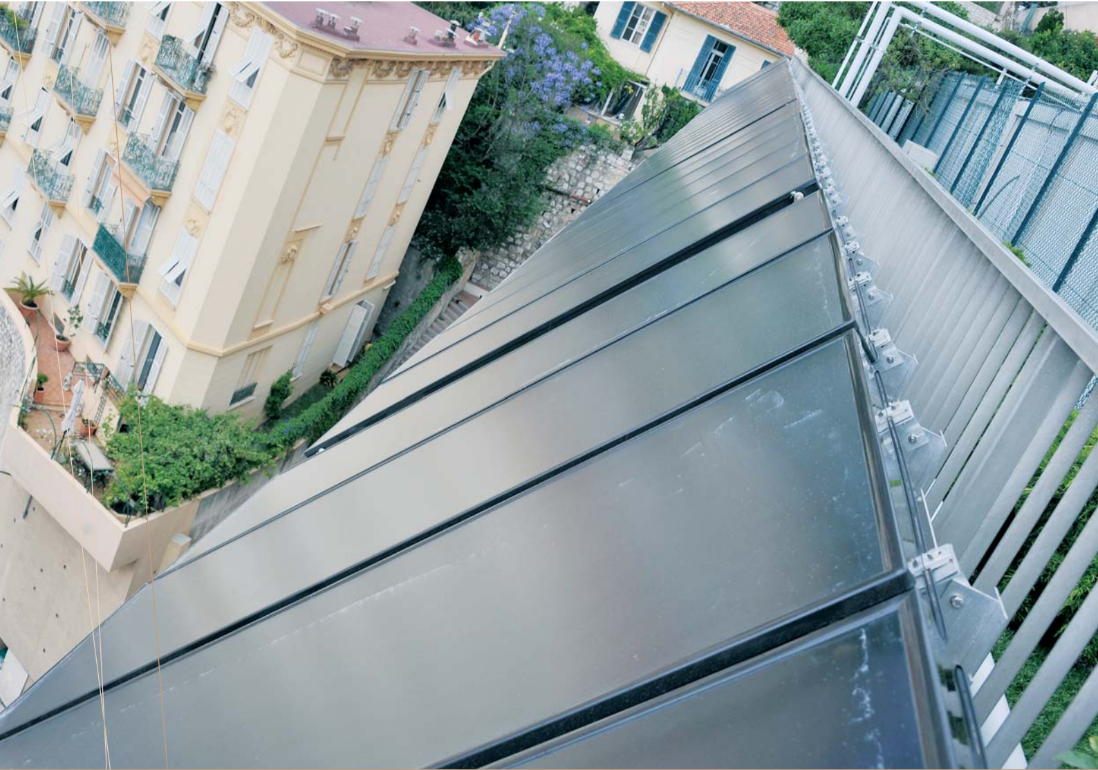
Solar panels on the Annonciade complex
